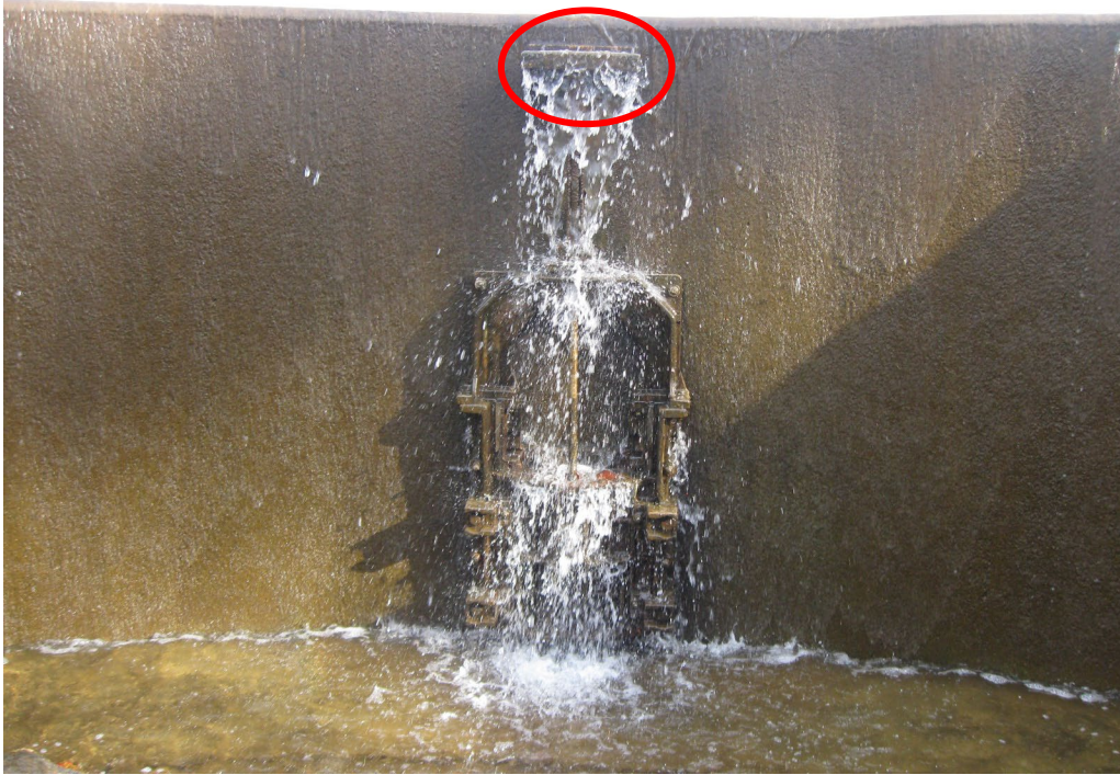
Photo No. 33: Closeup of the low-level outlet sluice gate. Note the deflection cover over the hydraulic operating cylinder.
