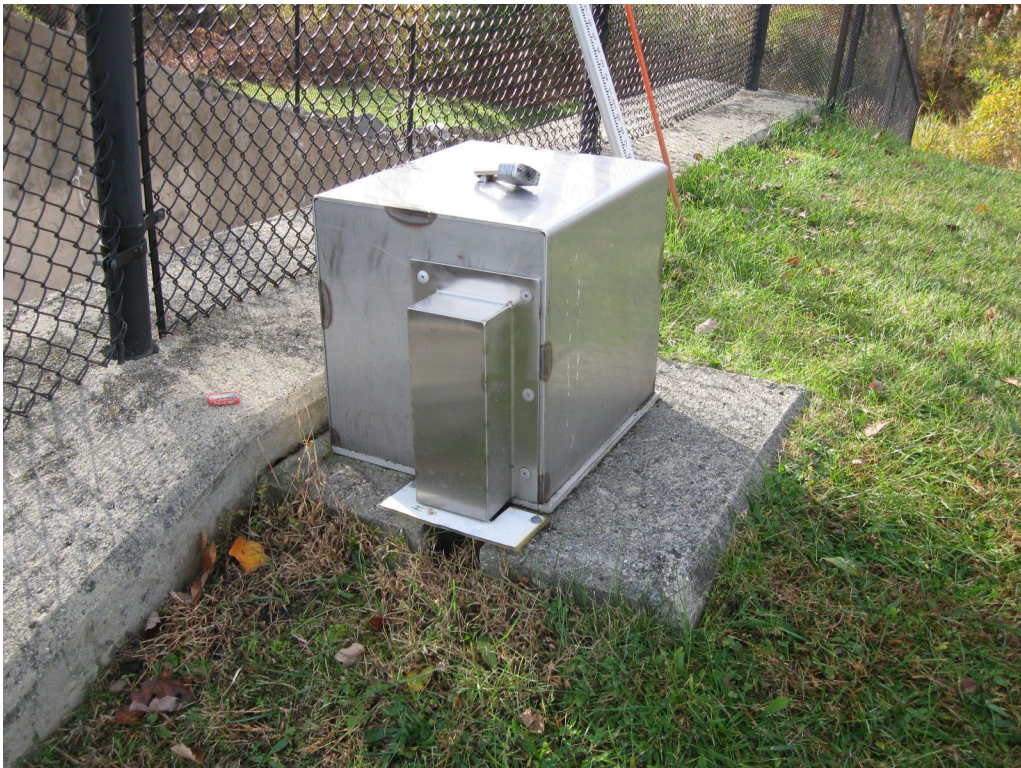
Photo No. 34: Hydraulic operator enclosure for the low-level outlet sluice gate.
