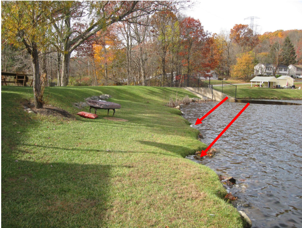
Photo No. 7: Left side upstream slope of the dam looking right toward the spillway. Note the scarping along the lake edge at the bench.
