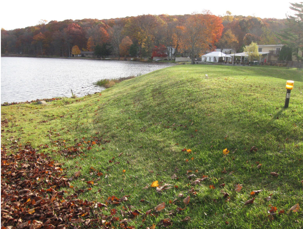
Photo No. 6: Right side upstream slope of the dam looking left toward the bend.
