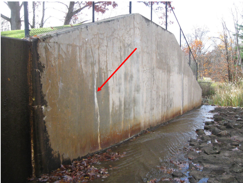
Photo No. 26: Left side spillway training wall looking downstream. Note the efflorescence and cracking in the wall.
