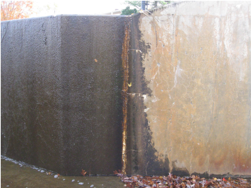
Photo No. 24: Joint between the spillway and the left side training wall. Note the the repaired joint material.
