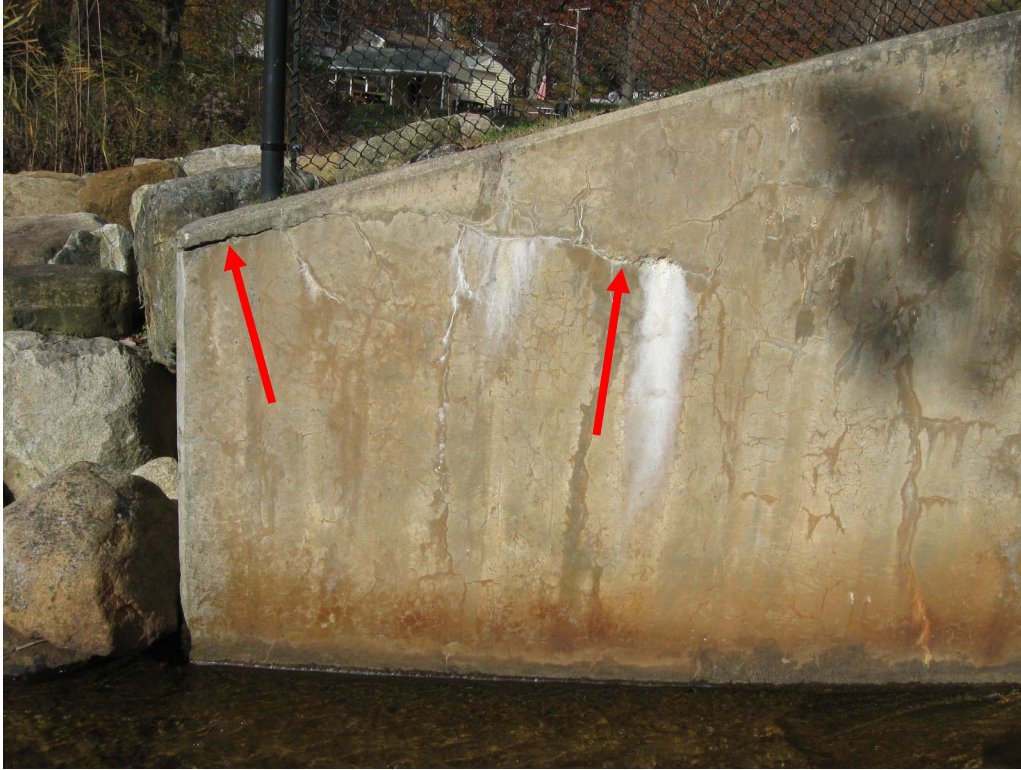
Photo No. 27: Closeup of 5-foot long horizontal crack in the downstream end of the right spillway training wall.
