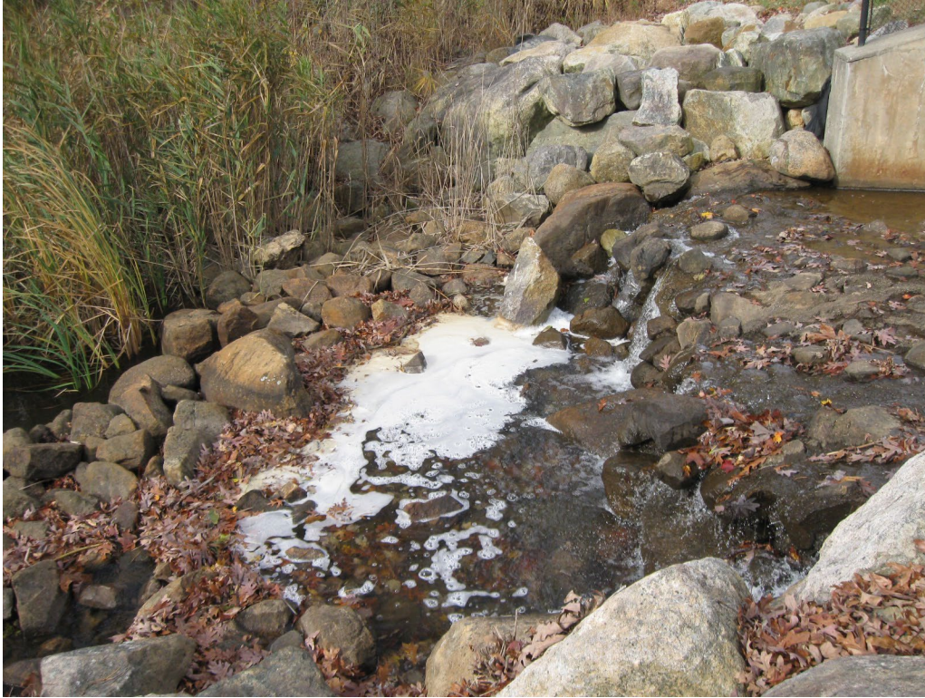
Photo No. 31: Downstream riprap apron looking right. Note that some riprap was added since the 2020 inspection.
