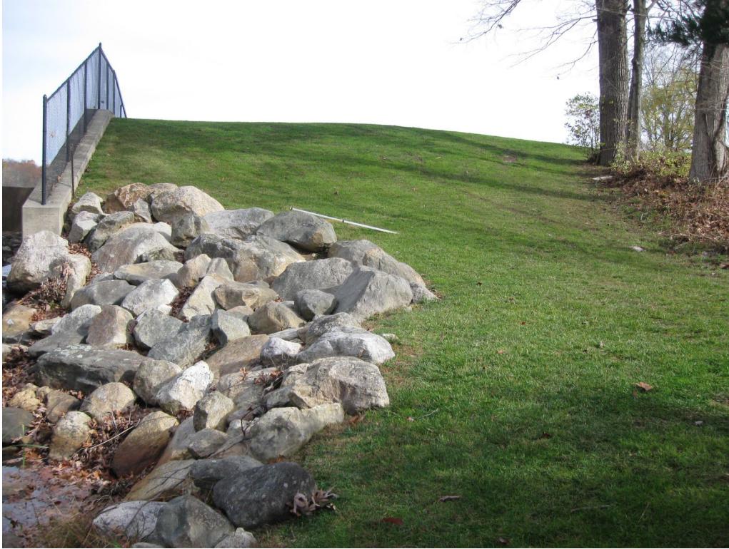
Photo No. 11: Left side downstream slope of the dam looking upstream from the toe.
