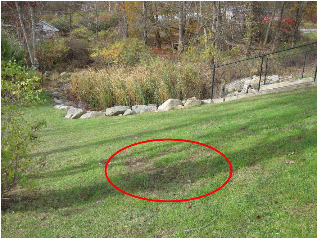
Photo No. 12: Left side downstream slope of the dam looking right toward the spillway. Note the area of sparse grass cover.
