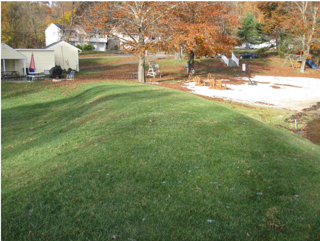
Photo No. 2: Right side dam crest looking right toward the right abutment.
