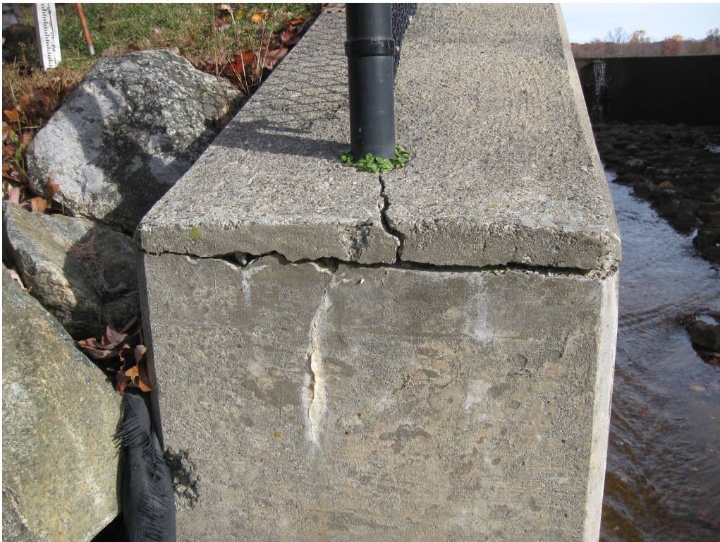
Photo No. 28: Closeup of horizontal crack in the top of the right training wall extending from the downstream end of the wall to the fence post.
