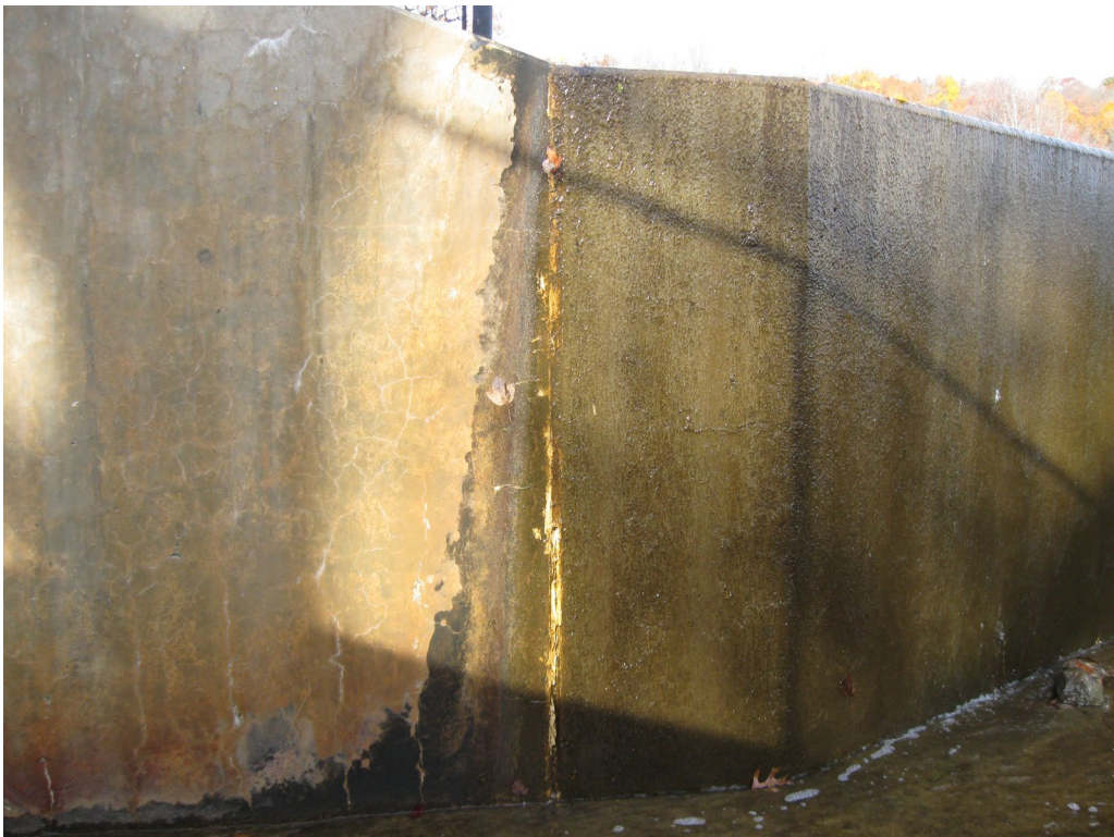
Photo No. 22: Joint between the spillway and the right side training wall. Note the the repaired joint material.
