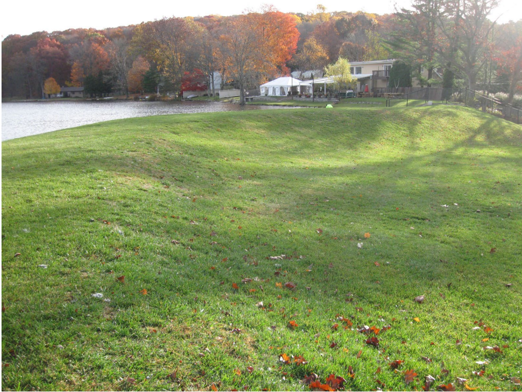
Photo No. 9: Right side downstream slope and toe of the dam looking left toward the spillway.
