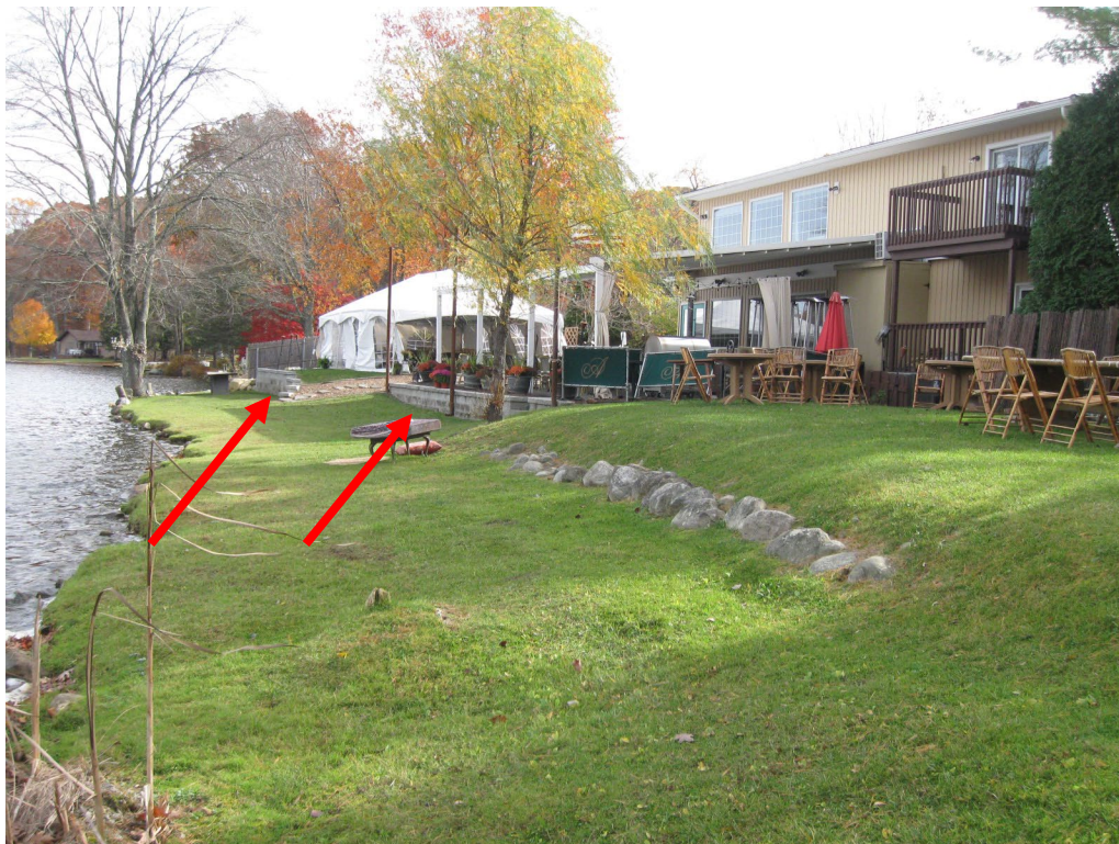
Photo No. 8: Left side upstream slope of the dam looking left along the restaurant. Note the segmental block retaining walls.
