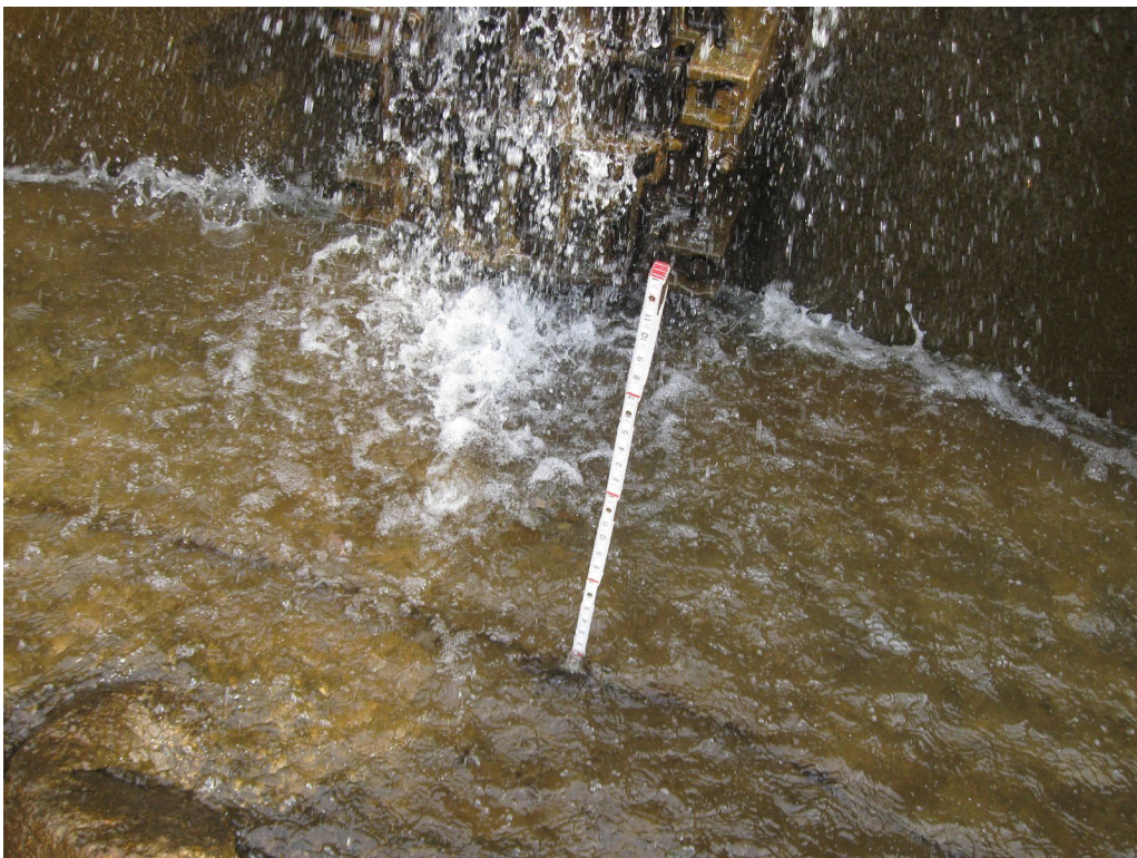
Photo No. 20: Closeup of a typical void between the spillway footing and the grouted riprap apron.
