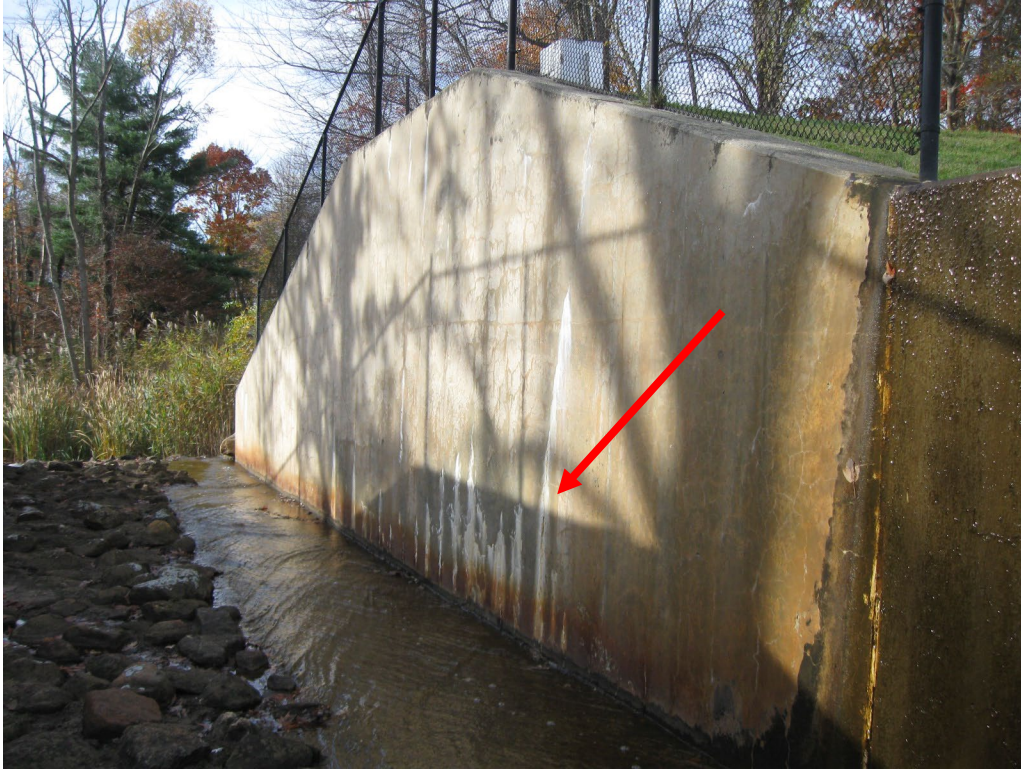
Photo No. 25: Right side spillway training wall looking downstream. Note the efflorescence and cracking in the wall.
