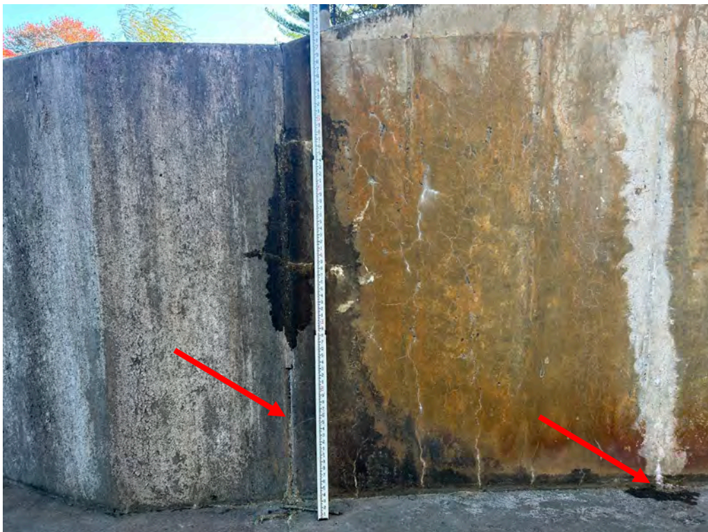
Photo No. 24: Joint between the spillway and the left side training wall. Note the the missing joint material. Also note the minor weep from the repaired crack in the bottom of the left training wall.
