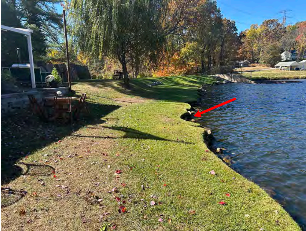
Photo No. 7: Left side upstream slope of the dam looking right toward the spillway. Note the scarping along the lake edge at the bench.
