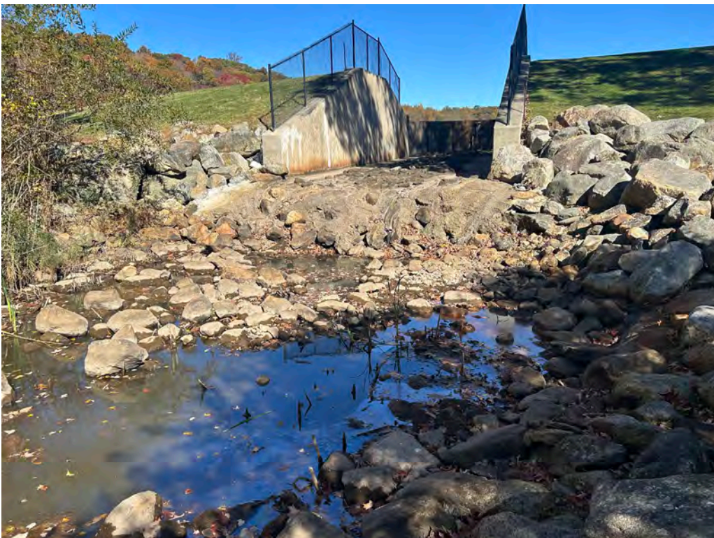
Photo No. 32: Downstream riprap apron looking upstream. Note the extension of the grouted riprap onto the apron since the 2022 inspection.
