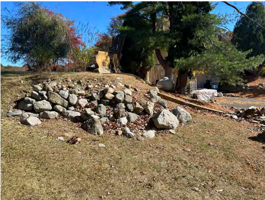
Photo No. 14: Closeup of the rock rubble wall on the left side downstream slope of the dam looking left toward the restaurant.
