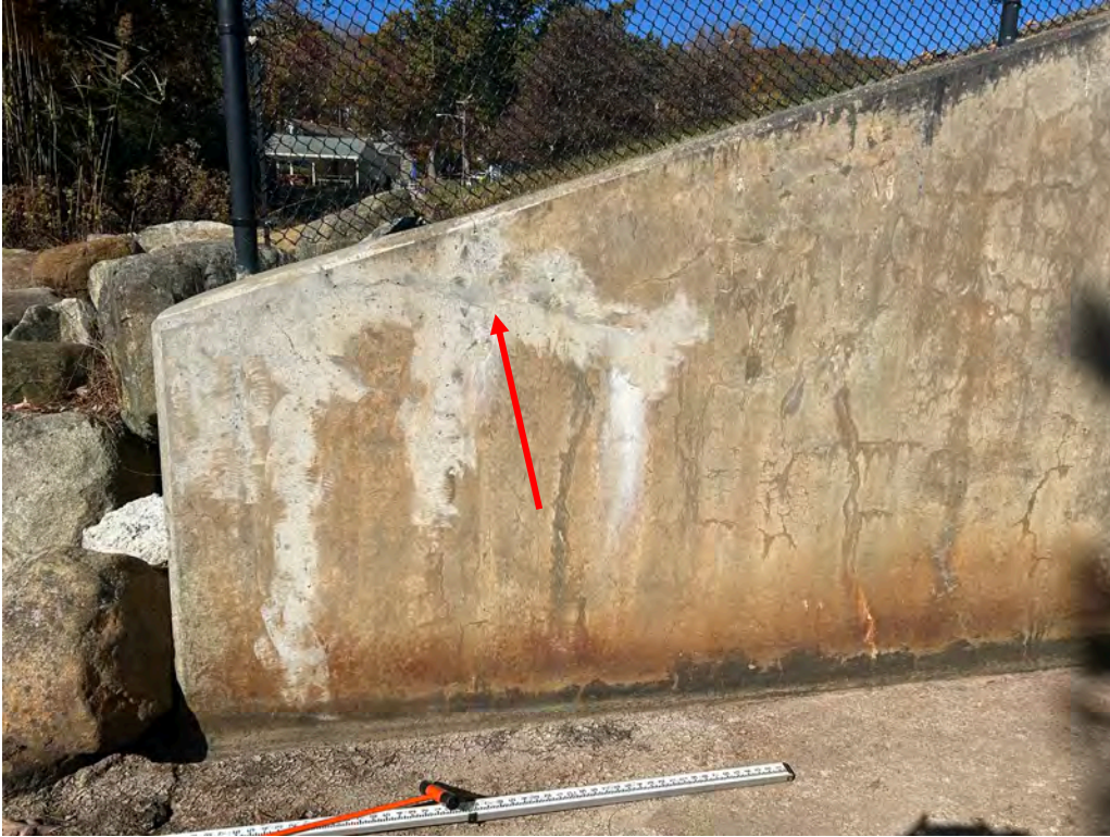
Photo No. 27: Downstream end of the right spillway training wall. Note that the 5-foot long horizontal crack was repaired.
