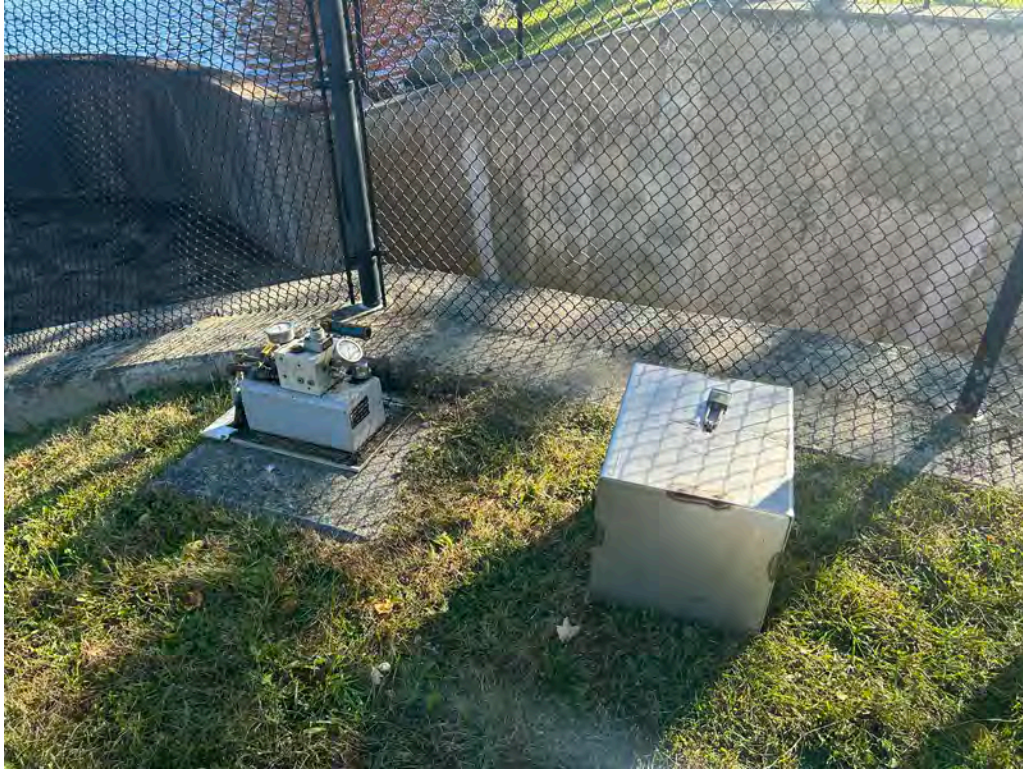
Photo No. 35: Hydraulic operator and enclosure for the low level outlet sluice gate.
