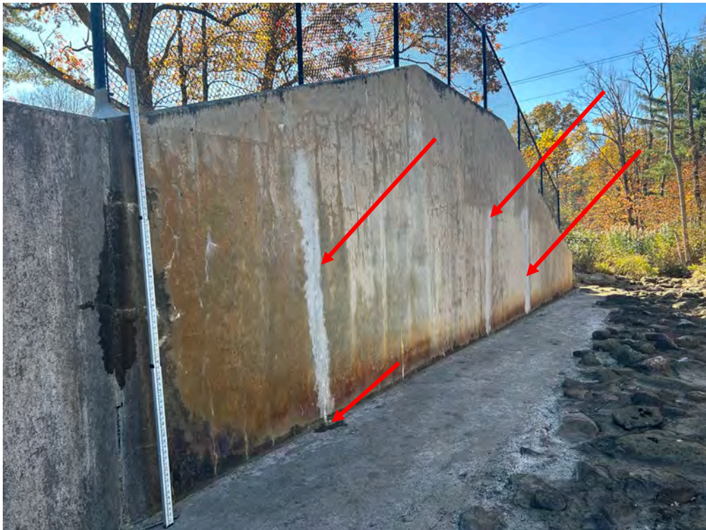
Photo No. 26: Left side spillway training wall looking downstream. Note the efflorescence and repaired cracks in the wall. Also note the minor weep from the repaired crack in the bottom of the left training wall.
