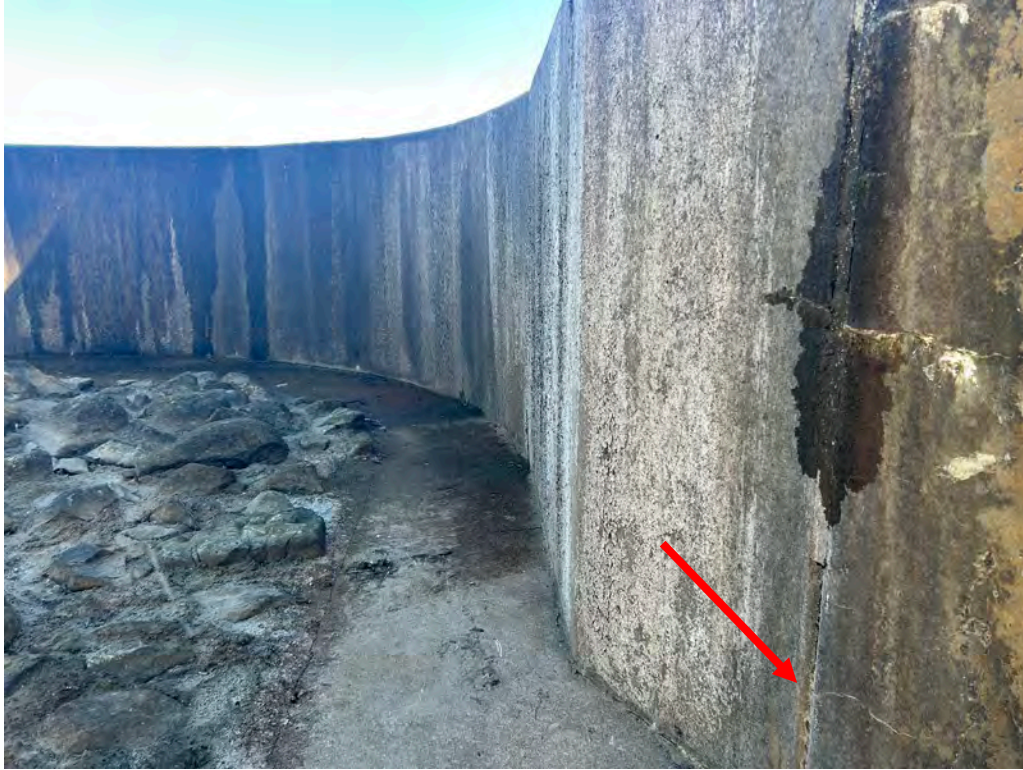
Photo No. 23: Left side downstream face of spillway looking upstream. Note the the missing joint material.
