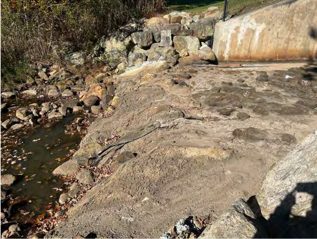
Photo No. 31: Downstream riprap apron looking right. Note the extension of the grouted riprap onto the apron since the 2022 inspection.
