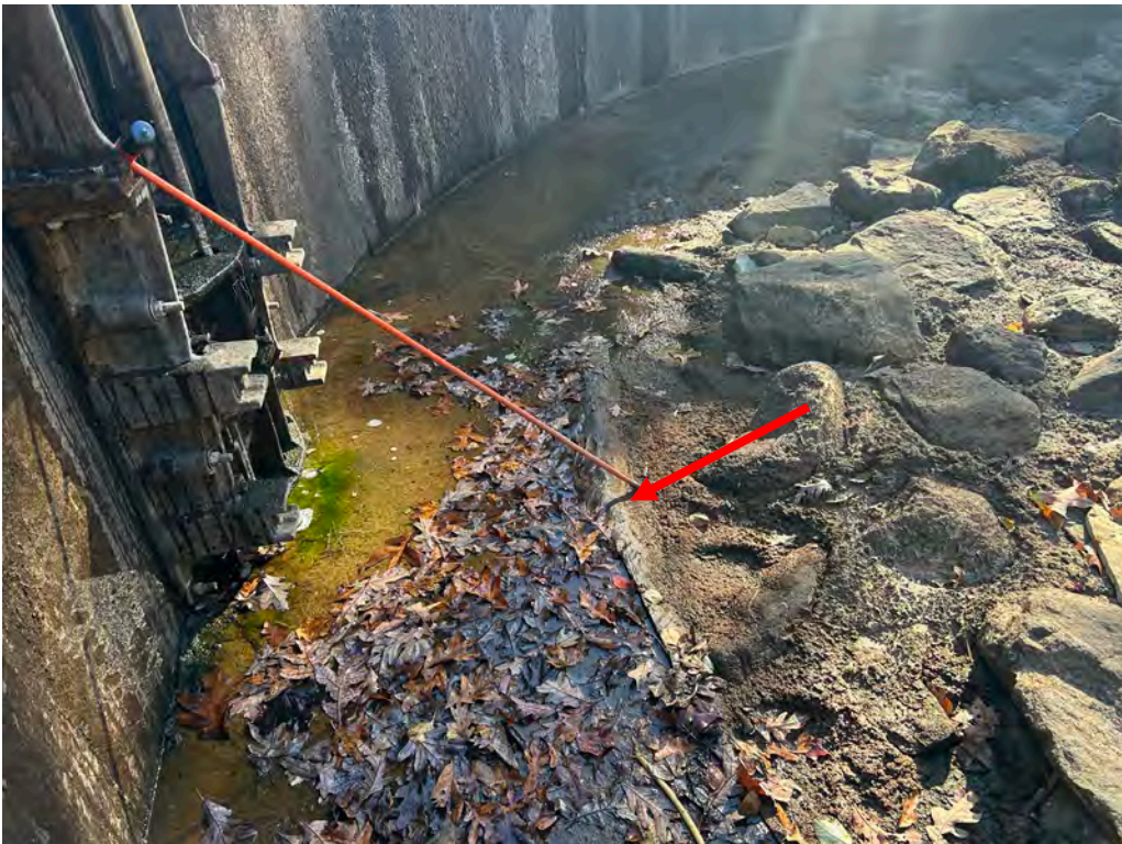
Photo No. 20: Repaired void between the spillway footing and the grouted riprap apron.
