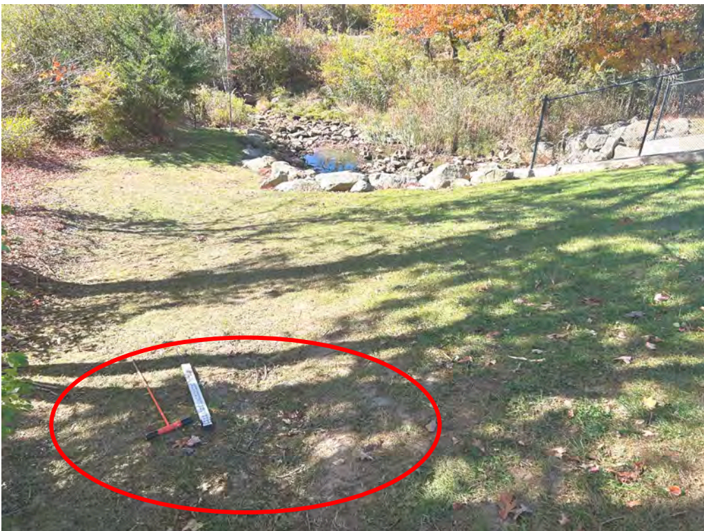
Photo No. 12: Left side downstream slope of the dam looking downstream. Note the area of minor erosion on the slope.
