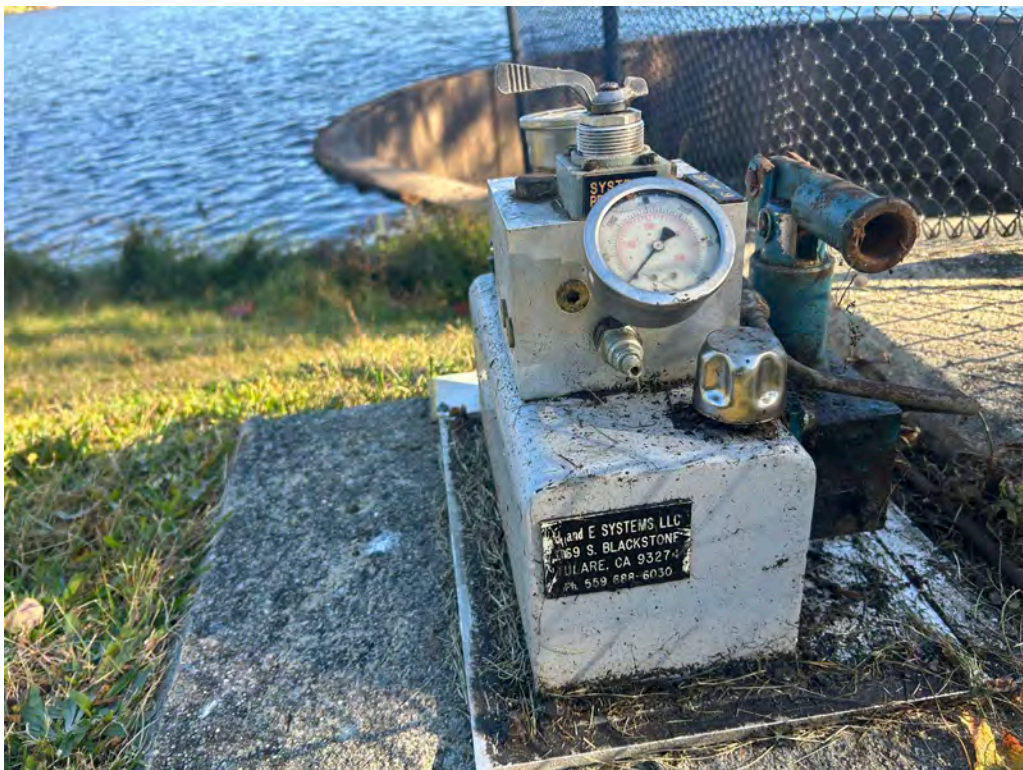
Photo No. 36: Closeup of the hydraulic operator for the low level outlet sluice gate.
