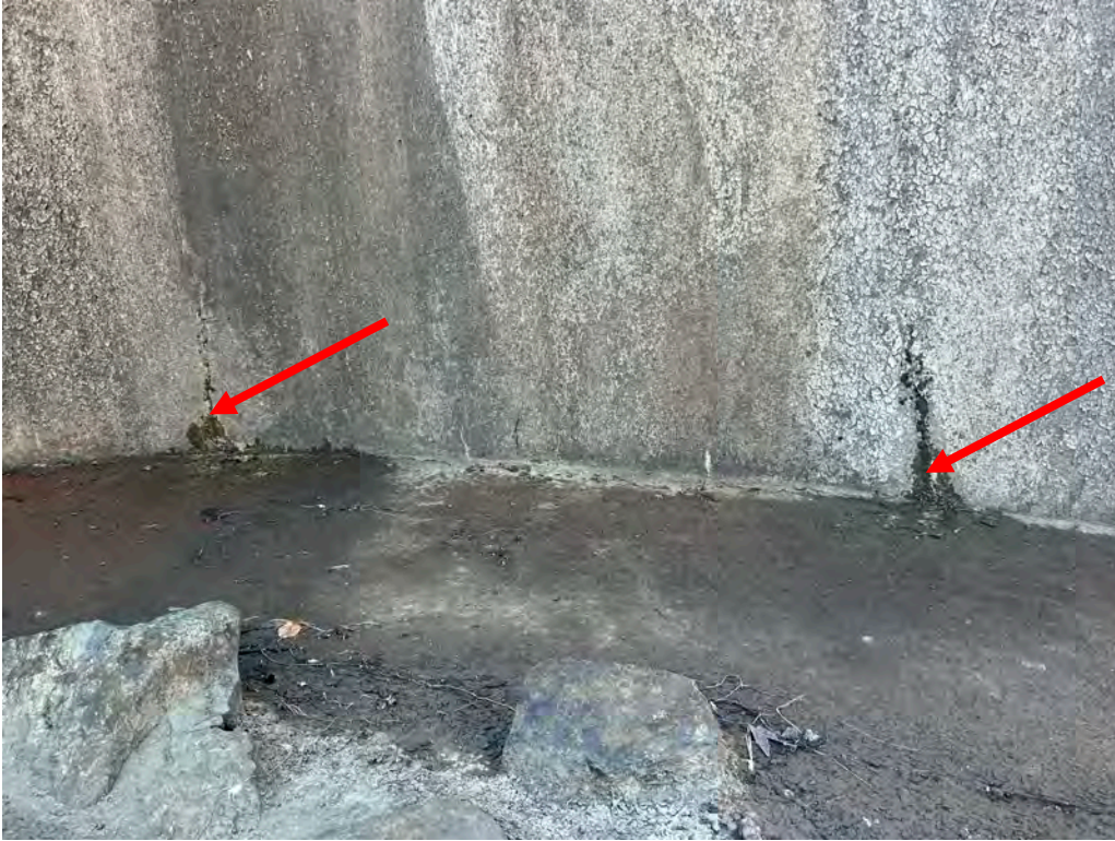
Photo No. 19: Minor weeps in the downstream face of spillway.
