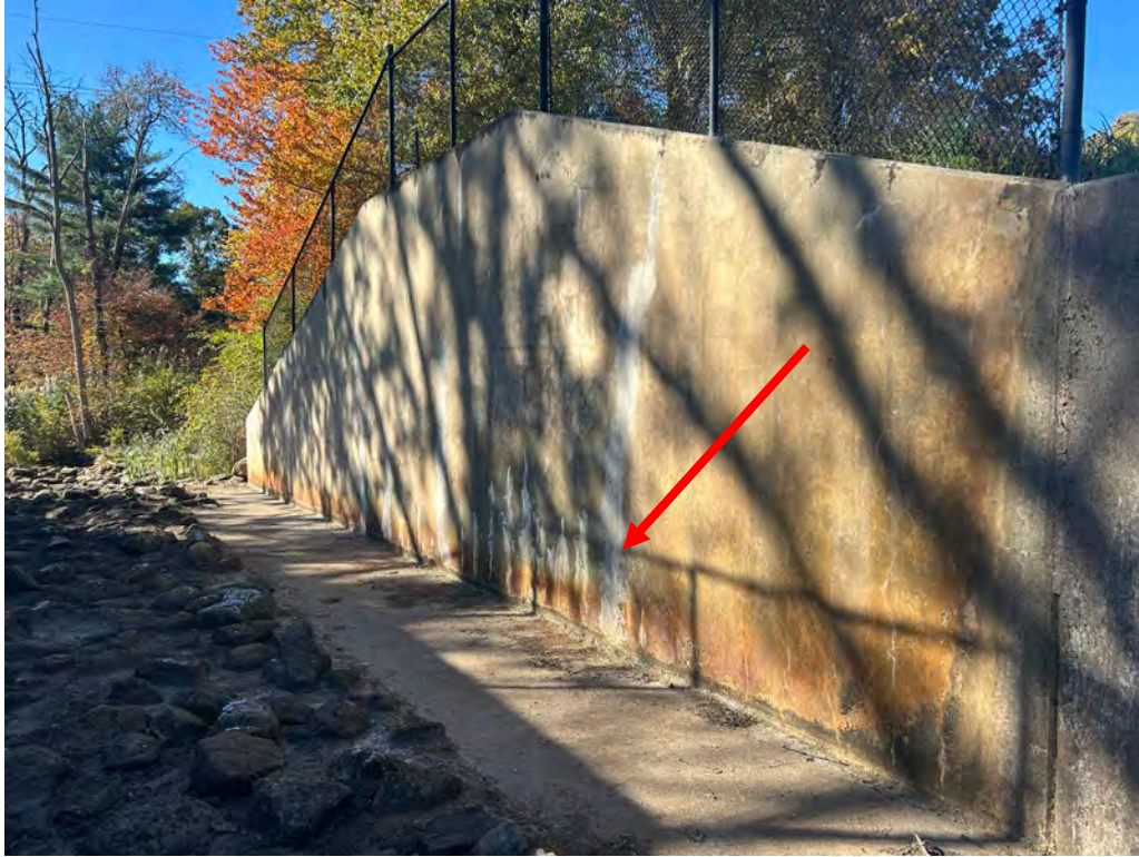
Photo No. 25: Right side spillway training wall looking downstream. Note the efflorescence and repaired cracks in the wall.
