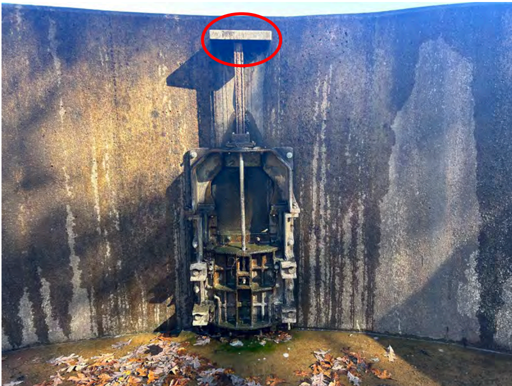
Photo No. 34: Closeup of the low level outlet sluice gate. Note the deflection cover over the hydraulic operating cylinder.
