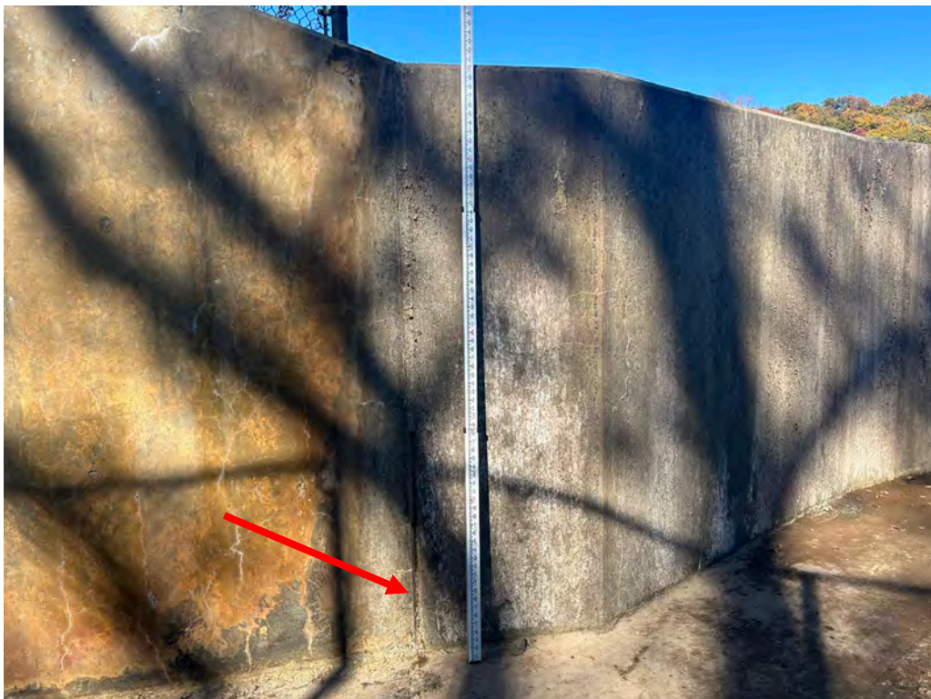
Photo No. 22: Joint between the spillway and the right side training wall. Note the the missing joint material.
