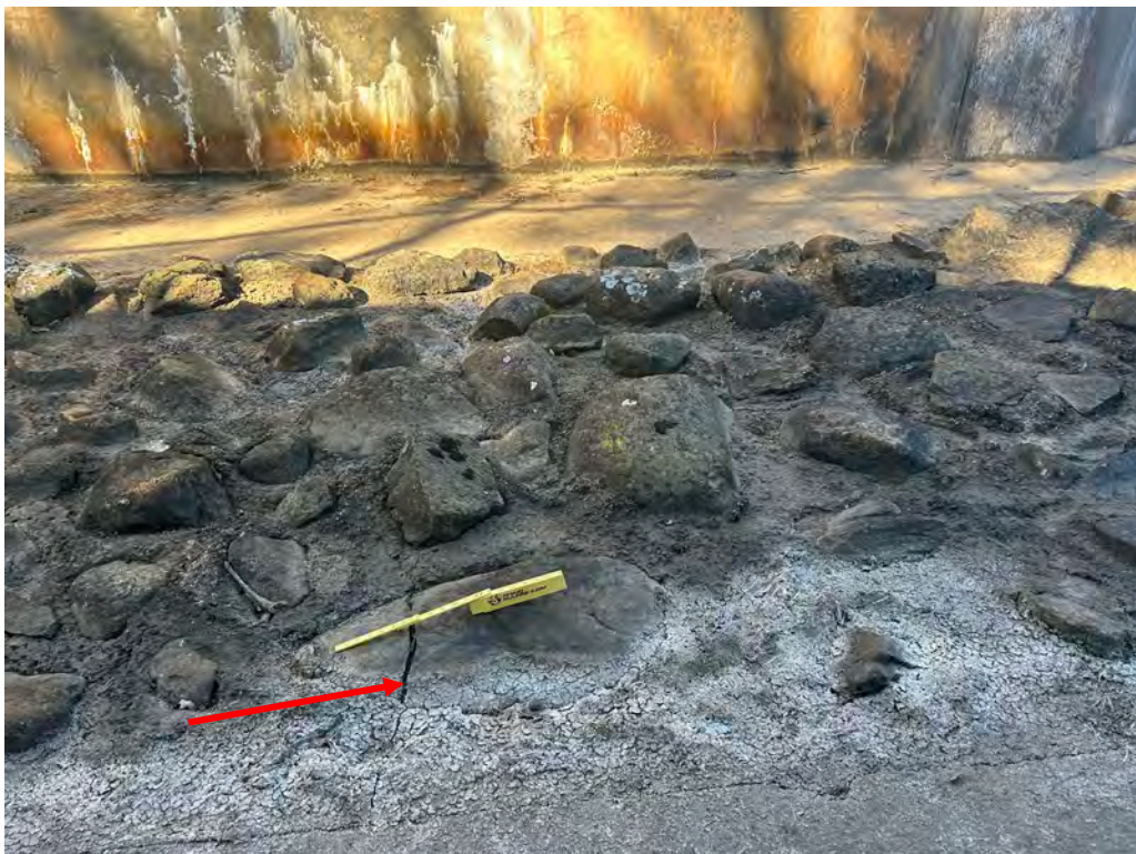
Photo No. 30: Crack across the grouted riprap discharge channel looking toward the right training wall.
