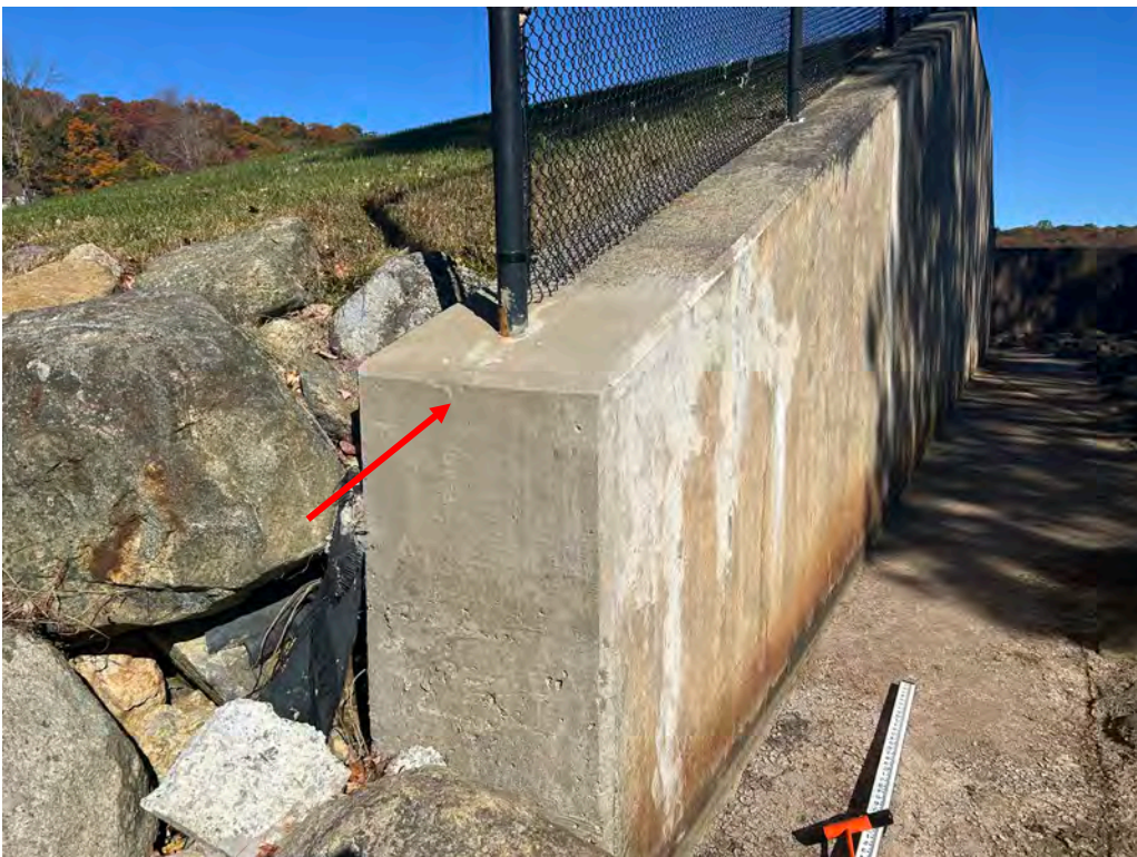
Photo No. 28: Top of the right training wall at the downstream end of the wall Note that the crack was repaired.
